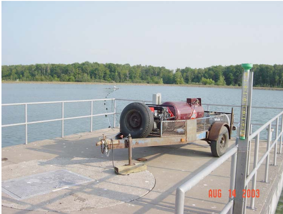
Figure 16 : Generator and Pump Trailer on boat dock for Test #3 at Isle.
