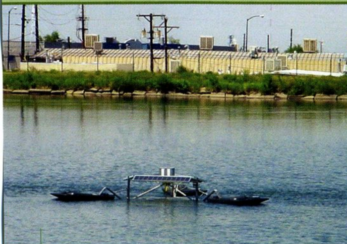
In June 2002, the City of Englewood, Colo., installed a SolarBee unit in its 80-million gal drinking water reservoir for blue-green algae control.
