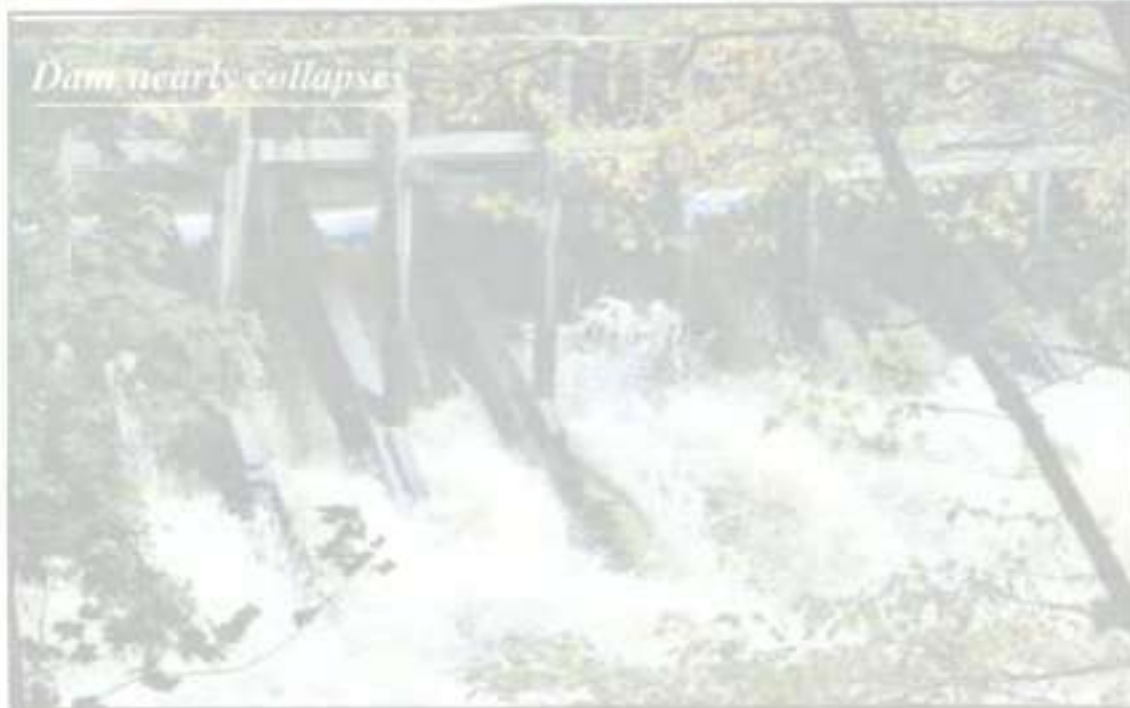
Near disaster. Water rushes over the Whittenton Dam on the Mill River in Taunton, Mass. recently. City officials were watching the 173-year-old wood dam carefully, fearing it might break and flood downtown Taunton with six feet of water. The dam has now been strengthened and repaired.
